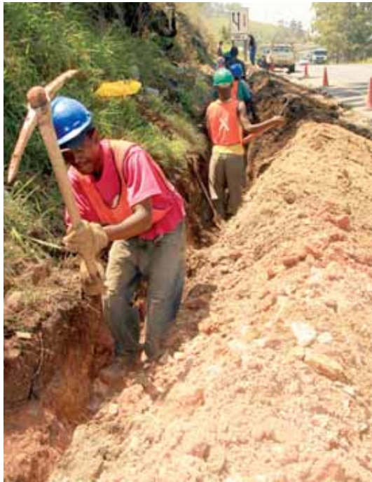
South Coast bulk pipeline
